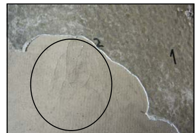
Figure 3 - Damage to surface of membrane with coating removed
