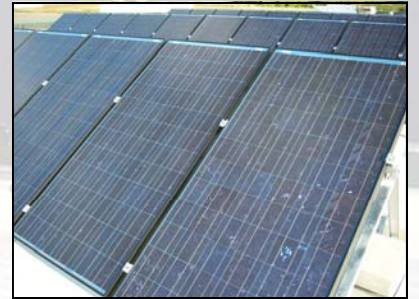
Rooftop Solar Panels
