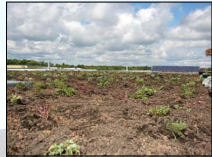
Prairie Green Roof System
