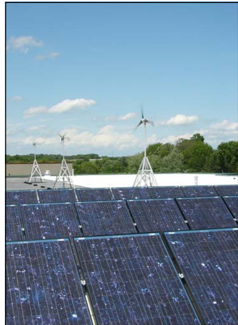
ERSystems Rooftop with Solar Panels and Wind Turbines
