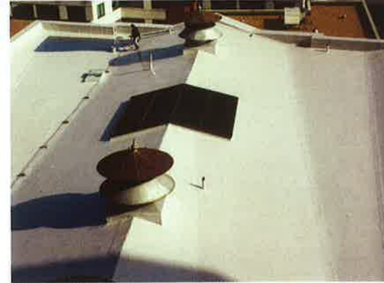
A 14-year-old built-up roof system before and after coating. The roof, coated in 1996, was recoated within the next five years to extend the coating's life.
